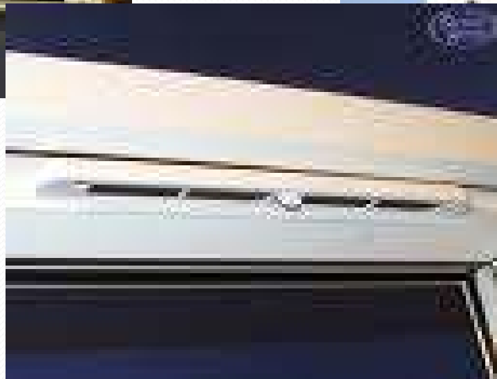
Whole building ventilation
